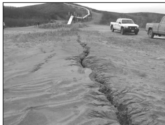
Figure 4. Surface evidence of liquefaction in the Delta River floodplain.
