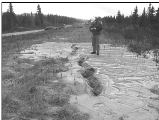
Figure 3. Surface evidence of liquefaction near Remote Gate Valve 91, south of Denali Fault.
