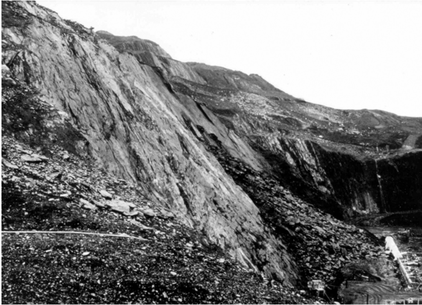
Figure 1. Failure of the PVR Slope in 1976
